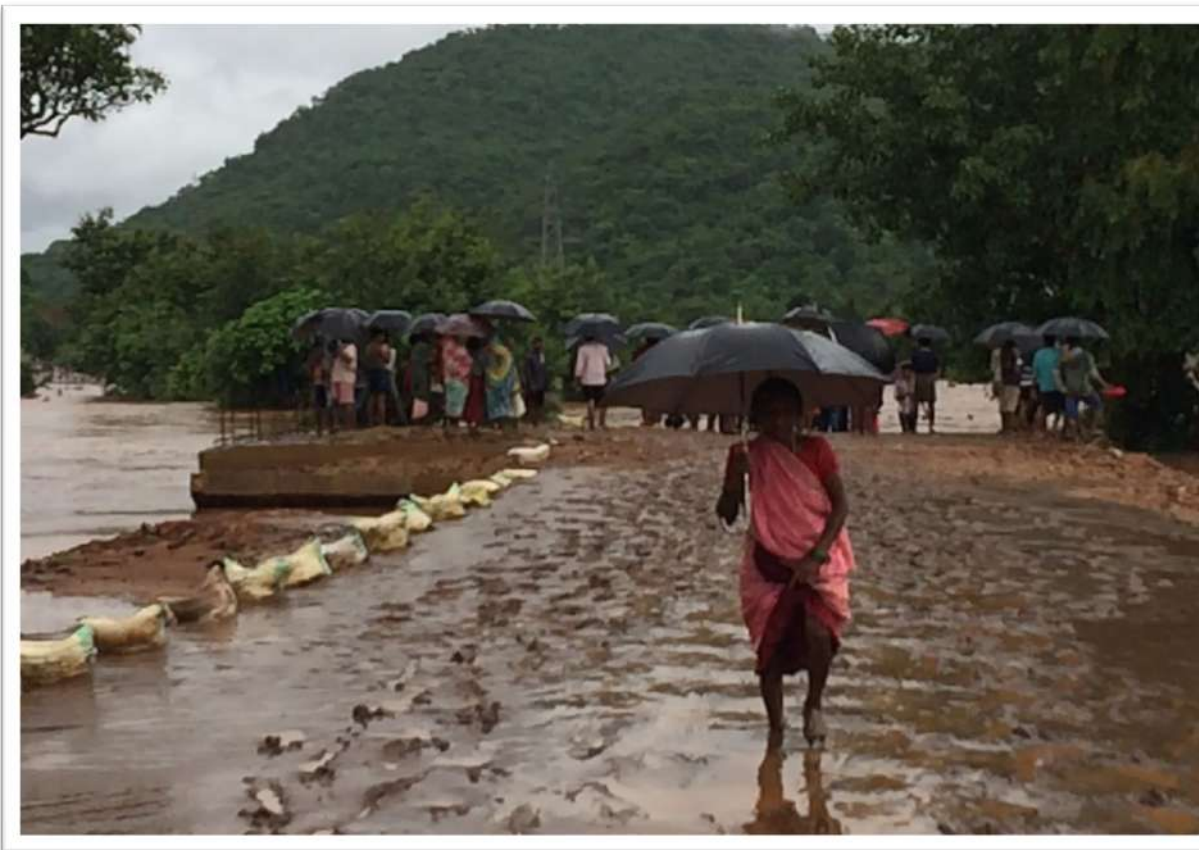
Pravatipur – Gunupur Road washed away
